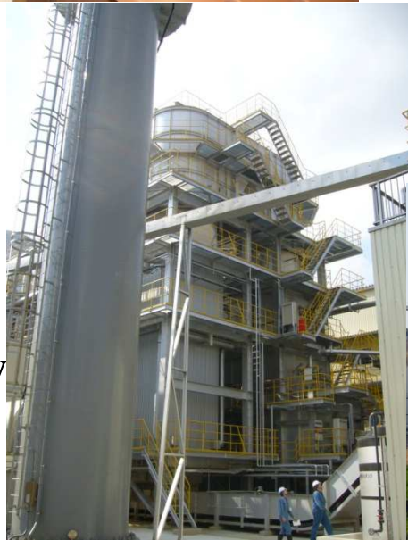
Incineration with Heat Recovery
