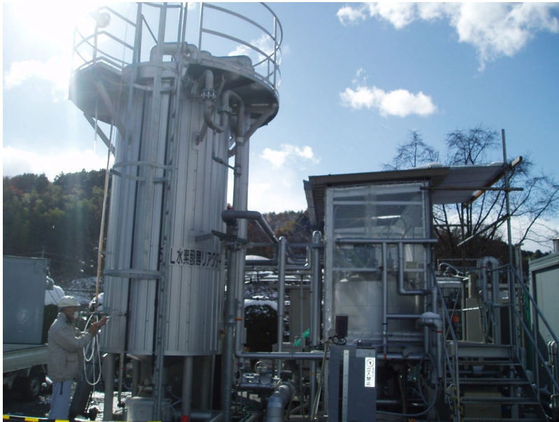
5m 3 -scale Hydrogen Fermenter
